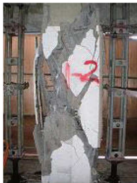
Photo1: Shear failure of a column of 5-story reinforced concrete building in Tokamachi city damaged during the 2004 Mid Niigata Prefecture Earthquake [6]
